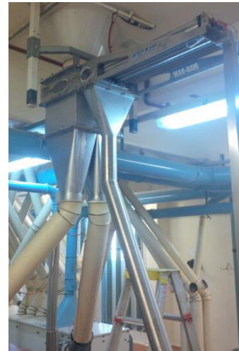
Example of contaminant discharge piped to a separate collection point.
