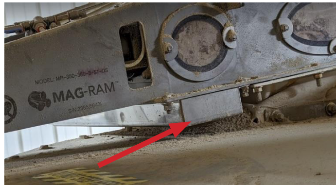
An example of an overloaded contaminants chamber
